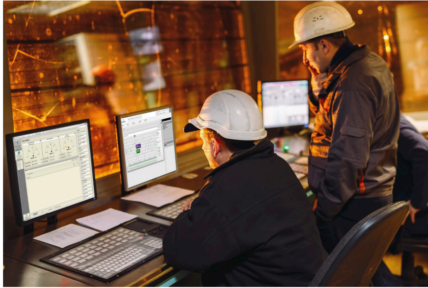
Figure 5. The ability to perform proof-tests remotely from the control room increases worker safety and efficiency.
