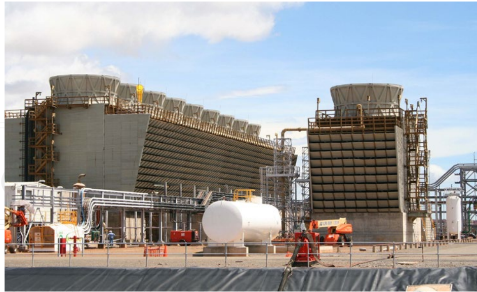
Figure 8: Cooling towers need monitoring because they have complex and often troublesome blower systems, in addition to fluid handling equipment.
