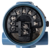
Figure 3-36 – Terminal Block Transient Suppressor
