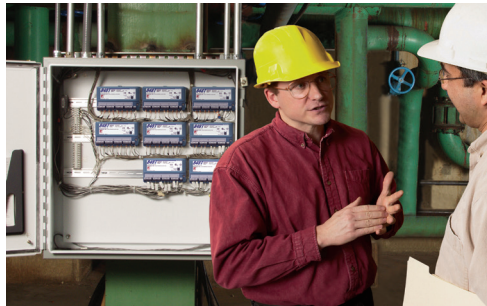
Figure 4-21 – High Density Field Mount Installation
