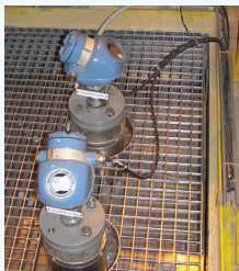
Picture 3.2 and 3.3: Two continuous measurements of the same type are used as the level sensors in the BPCS and the safety layer (left: radar level gauges, right: guided wave radar level transmitters)
