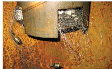
Picture 3.1: Unreliable mechanical level transmitter (servo type)
