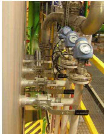
Figure 1. Three Rosemount 5301 Guided Wave Radars used for condenser level control.
