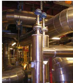
Figure 3. Reliable level measurement on this pre-heater tank provides improved process stability.
