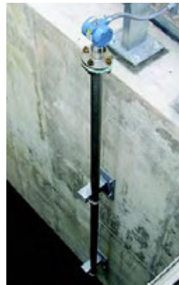
Guided Wave Radar Installed
