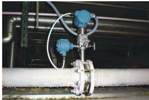
Figure 4.4: A Rosemount Compact Annubar™ Flow Meter installed in a natural gas line at a pulp and paper mill.
