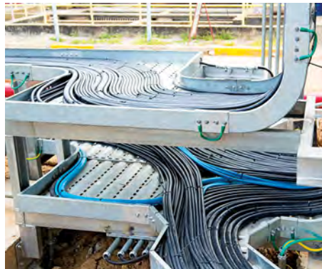
Figure 10.17: Conduit and cable tray.
