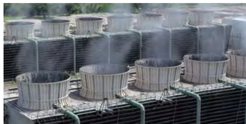
Figure 5.2: An industrial cooling tower, which uses evaporation of water to remove large amounts of heat from an industrial process.
