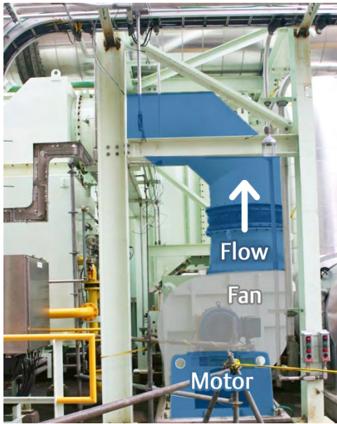
Figure 4.7: A boiler forced-draft fan for combustion air flow.
