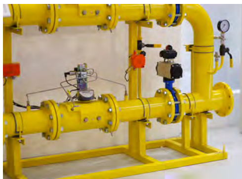
Figure 4.12: A furnace fuel control skid.
