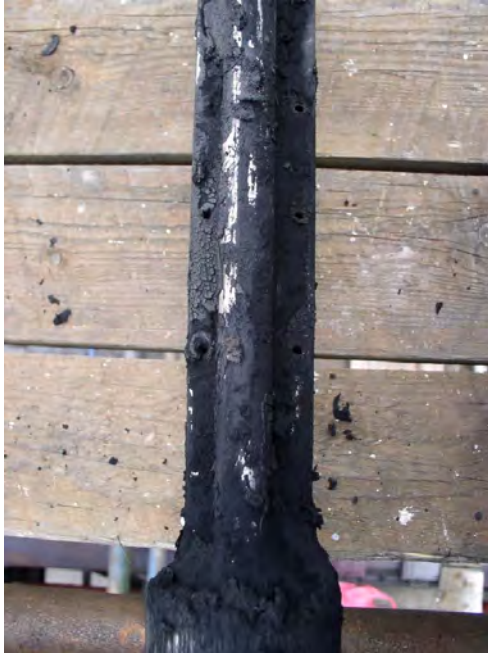
Figure 10.44: Close up of the solids buildup on the base of the Stack Annubar sensor exterior. Required maintenance is needed to clean the sensor periodically.
