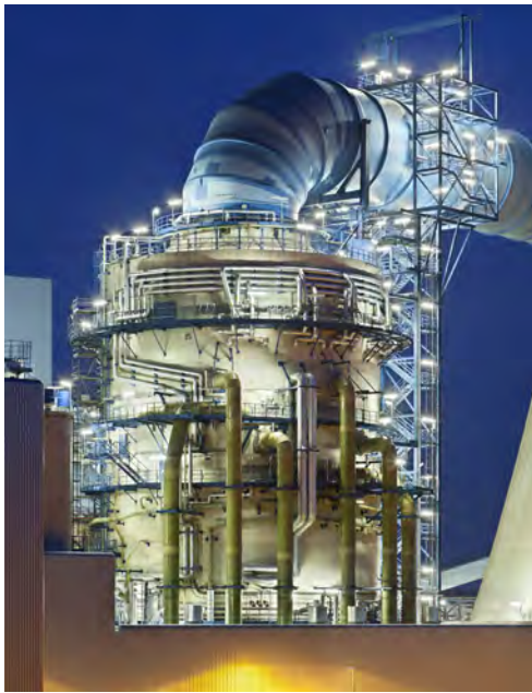
Figure 4.10: A utility scrubber for emissions reduction.
