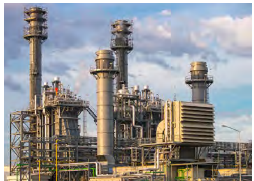
Figure 4.8: A combined cycle power plant with a large combustion air intake.
