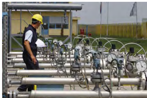
Figure 5.9: A midstream flow metering and regulation station.
