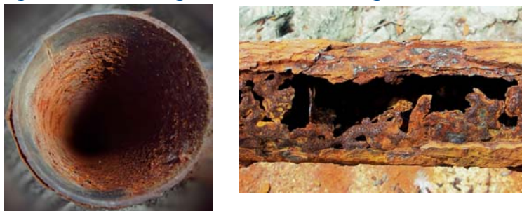
Figure 1. Boiler Scaling and Corrosion Resulting from Imbalanced Water pH
