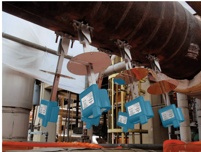
Figure 6. Array of Wireless Ultrasonic Sensors
