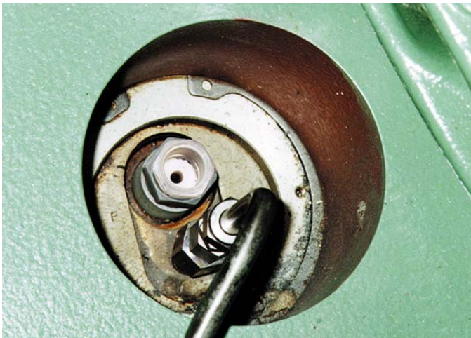
Cooper-Champion RW80N after experiencing Insulator break-up during operation.
